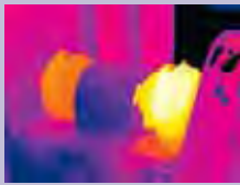
Overheating bearing cap
