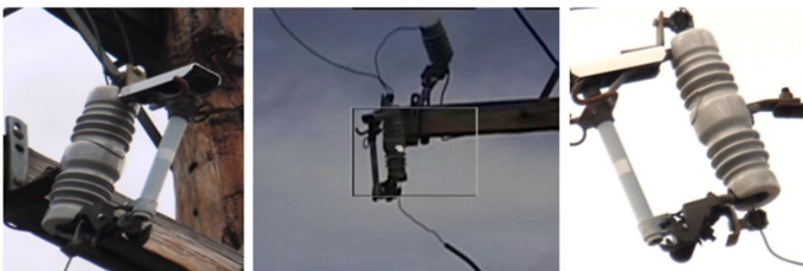
Figure 7: Cracked Cutout Insulator
