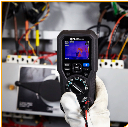
Thermal scan of an electrical panel
