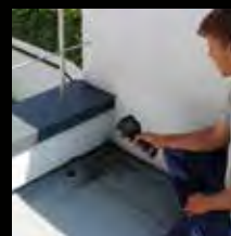
Discover leaks in roofs
